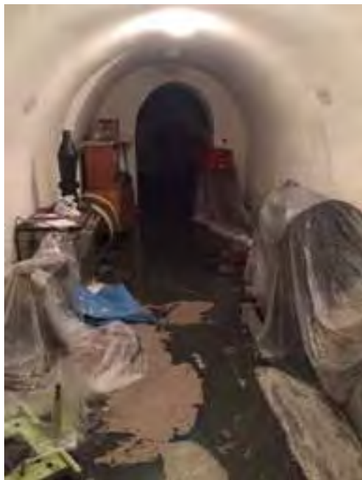
Flooding of the collection storage in the basement with waste water, 30/05/2018
